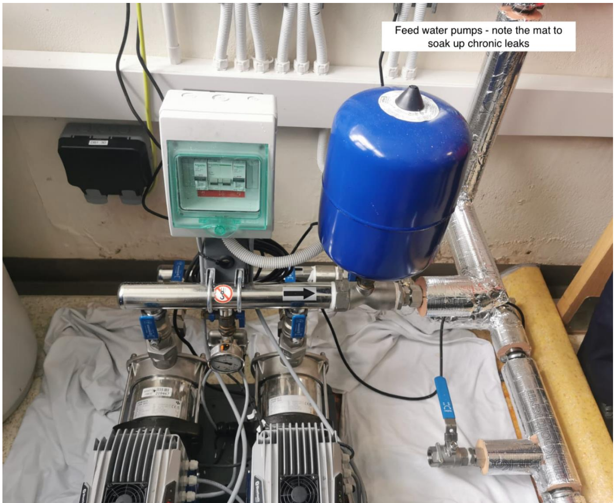
Figure 5 Photo of the feed water pumps in Bedford renal unit
